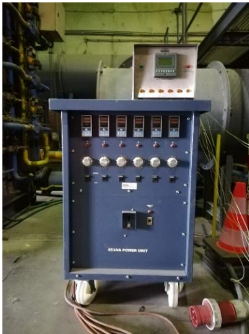
(a) 65kVA transformer unit
