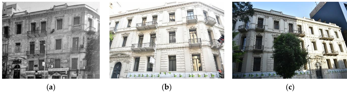
Figure 7. (a) Main façade before retrofitting scenarios (b) Main façade after retrofitting scenarios (first author’s Ph.D. research); (c) Another façade after retrofitting scenarios (first author’s Ph.D. research).
