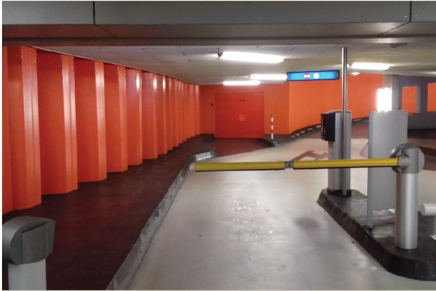
Figure 1. Walls in an underground car park made of unprotected steel sheet piles [1]
