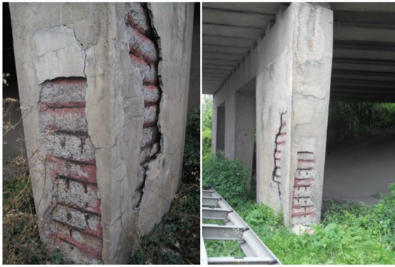
(a) Bridge piers with advanced corrosion (photos courtesy of Service Public de Wallonie)
