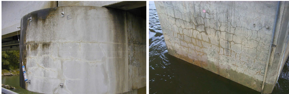
Figure 2.1: Examples of 2 different bridges in France that underwent sulfate attack. The damage appeared as a network of widely-spaced multidirectional cracks, only at places that were accessible by water. From Divet et al. [79].
