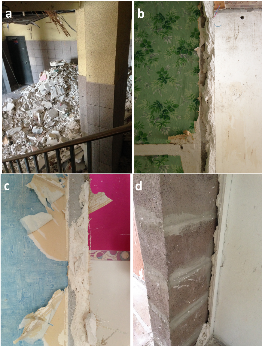
Figure 3.2: Plaster is being collected before demolition (a) of an apartment building, but gypsum residues are still present on walls (b-d) and will end up in recycled aggregates.
