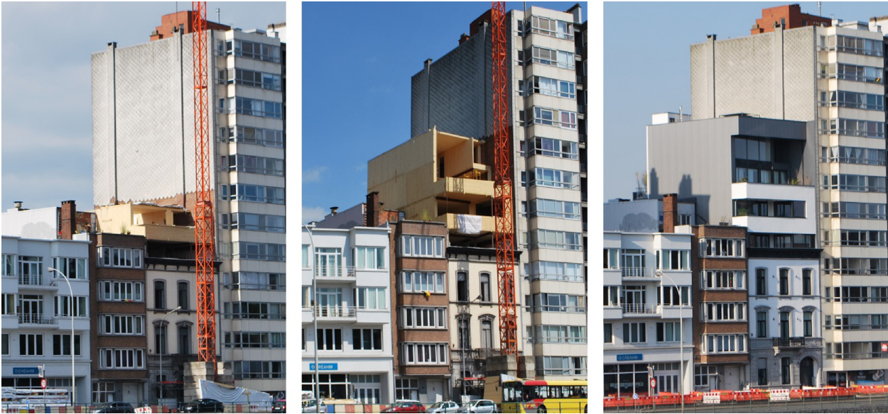
Fig. 1. An example of a roof stacking over an existing rooftop.
