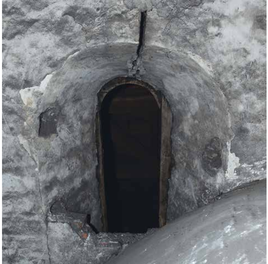
Fig. 7.7. Romanesque window, interior view. North wall, bay 3. Photo: K. Keutgens, B. Delmotte and P. Duerinck
