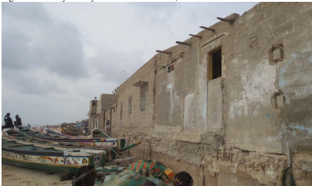
Figure 2: Partially destroyed home in Guet Ndar, Saint-Louis
