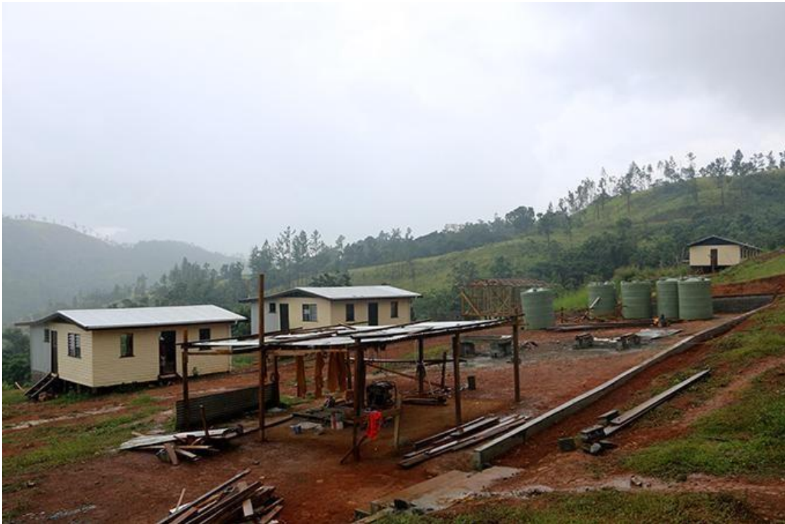
Figure 61: Tukuraki relocation site; the land of the Mataqali Yalimara/ Tokatoka Navuti. (Photo: Julie Cleaver/PMC)
