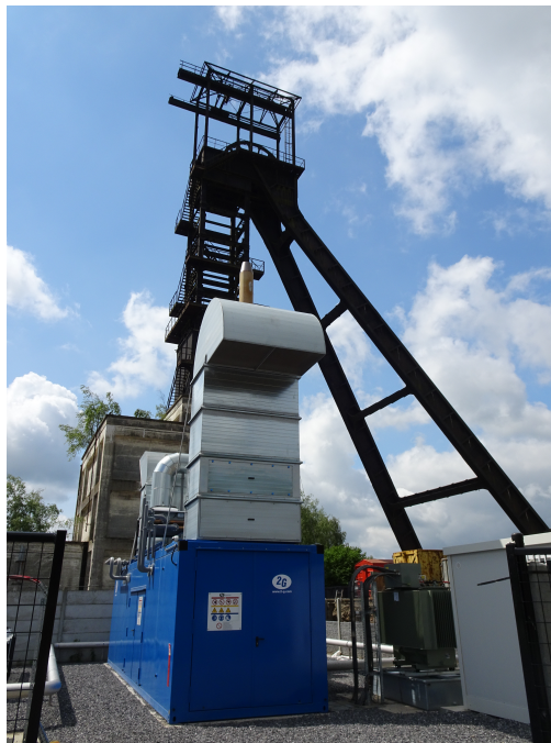
Figure I–16 – One of the engines generating 1.5MW at the foot of the headframe from an abandoned coal mine in Anderlues (Belgium). Photo taken on 06/06/2019.
