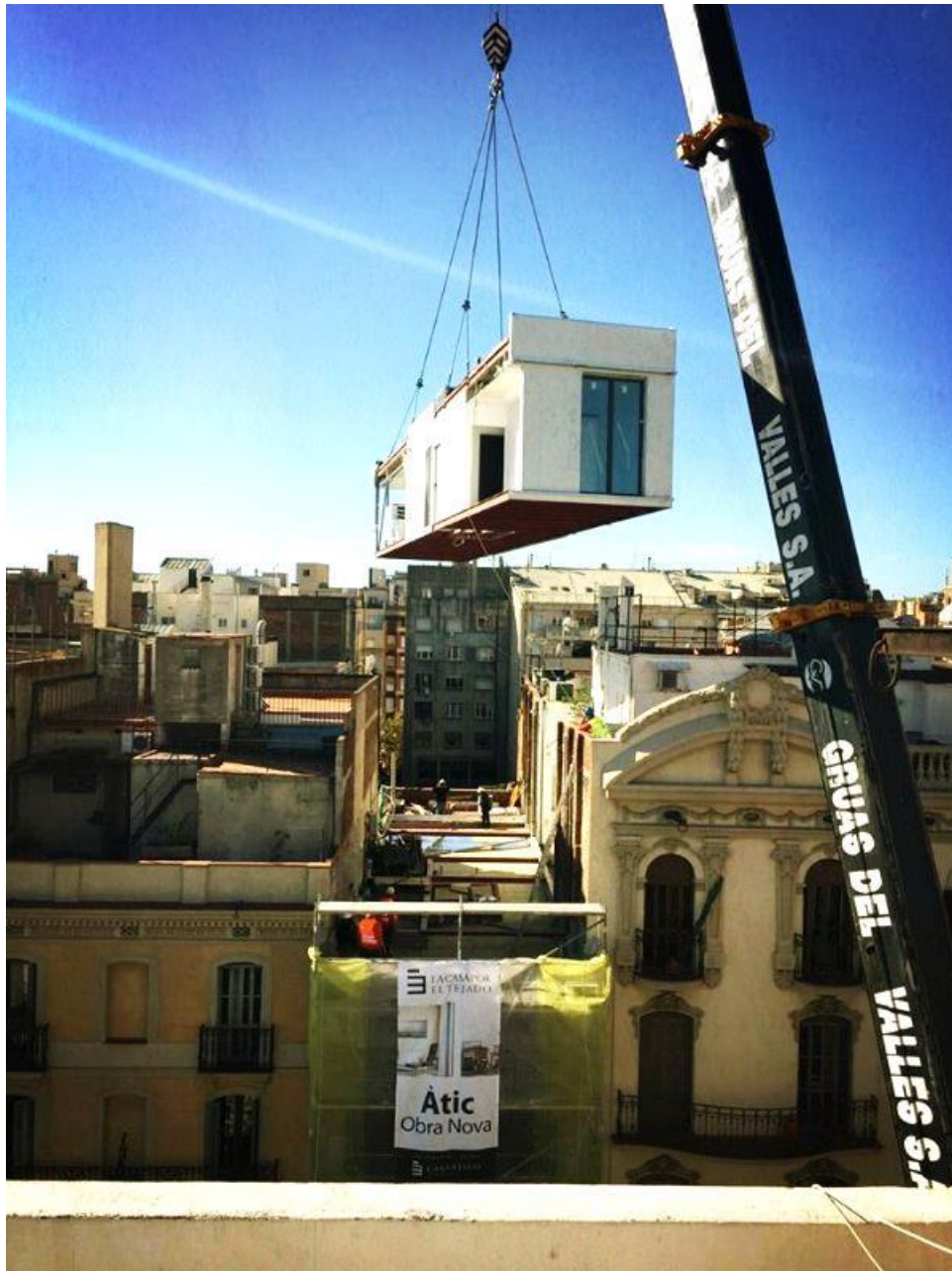
Figure 3-6: Roof stacking modular construction using large crane to lift a 12 meter length module in Barcelona, Spain © La Casa Por El Tejado
