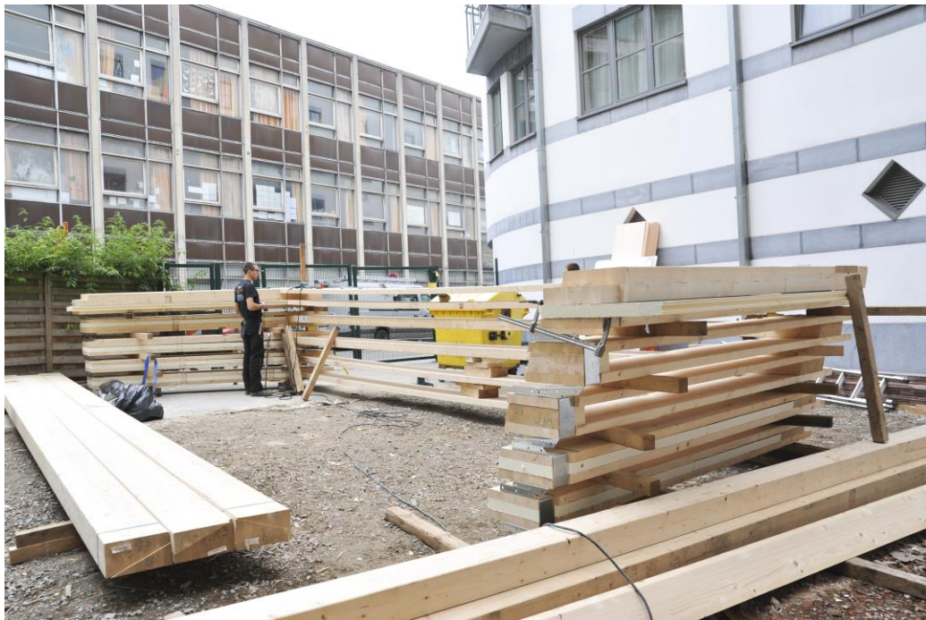
Figure 3-8: Roof stacking onsite elements' assembly (1D) using the existing courtyard of the building in Brussels, Belgium © Antoine Galand
