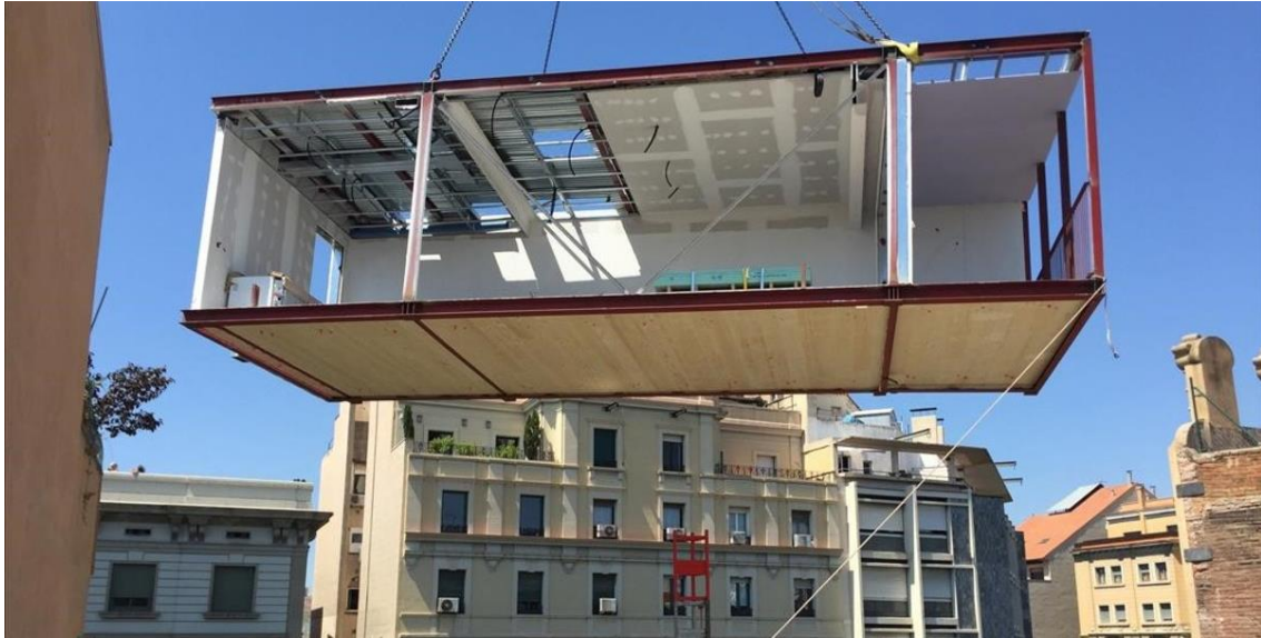
Figure 1-3: Lifting 3D modules over the rooftop in Barcelona © La Casa Por El Tejado
