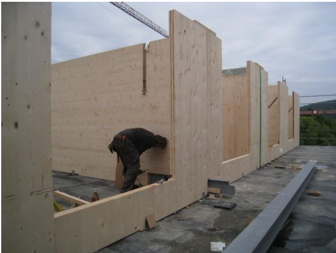
Figure 3-7: Roof stacking construction using CLT panels subjected directly on the rooftop at Kierling, Austria © Georg Reinberg
