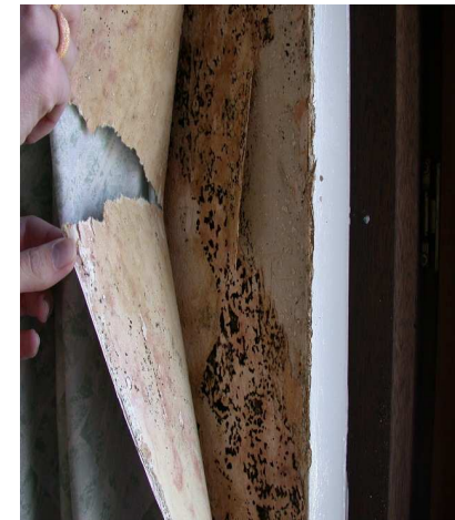
Detection of moulds in buildings
