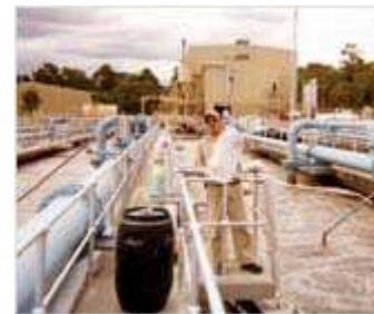
Waste water treatment
