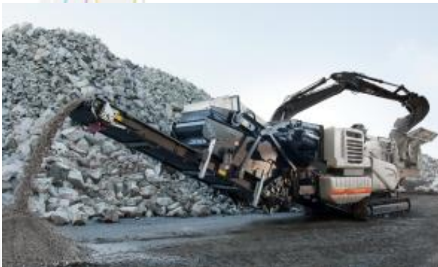
Mobile crusher Metso LT12113 250 t/h - 115 m 3 /h ; 1x /year (on-site storage of waste)
