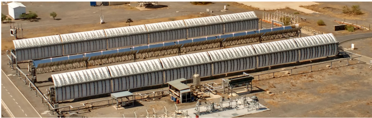
Fig. 3. Aerial view of the HTF loop at PSA, Almería.
