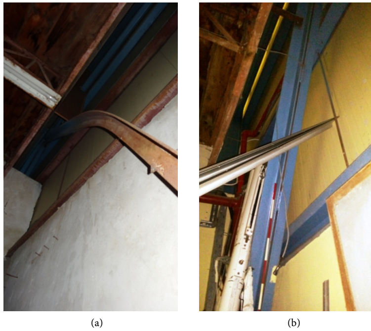
Figure 3. Vertical A-type bracing on the southern section of the building: (a) the corroded portion with major second-order deformation and (b) the undamaged portion.
