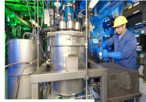
Bayer pilot plant
