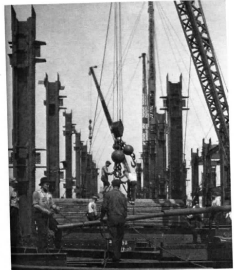
This derrick gang is moving a heavy load of planks while men in the foreground extend the bull stick of the derrick for greater leverage. Opposite, another connector goes aloft.
