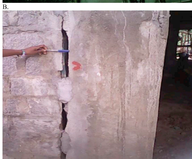
Fig. 2. A. Fissuring on the environment building induced by the construction of a 7 floors building in Behoririka (location cf. Fig. 1-C). B. Fissuring in relation to a punching failure in the foundation of a 3 floors building in Ambanidia-Ankazotokana (location cf. Fig. 1-C).
