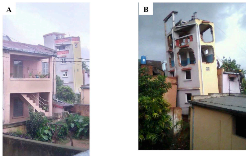
Fig. 11. Building demolition at risk of collapse in Antananarivo. Top: fire fighter operations statistics for January 2018 - (Source: Fire fighters). Bottom: A. Differential settlement of an R + 3 house foundation in Anjanahary II district O - 30th December 2017. B: Demolition of this house by firefighters to avoid collapse on surrounding environment (beginning of the year).
