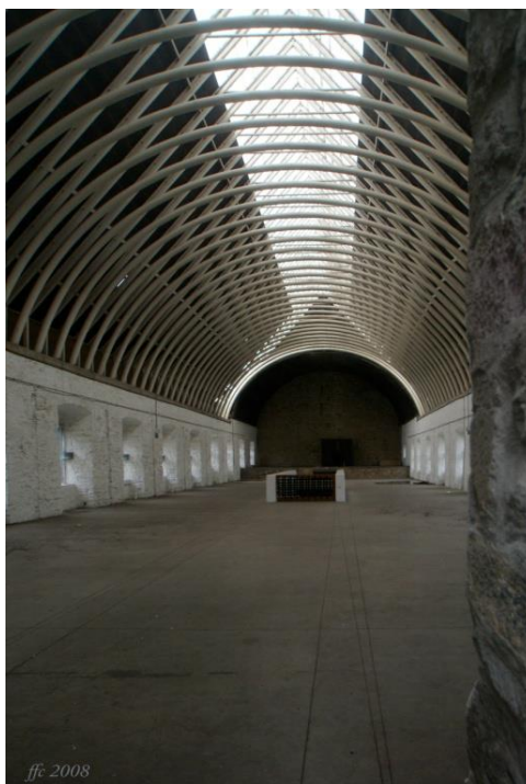
Fig. 2 The restoration architects, Moreau & Coyette, designed a new steel frame in accordance of 13th century barrel vault shape and measurements © Flamenc 2008 (under GFDL)
