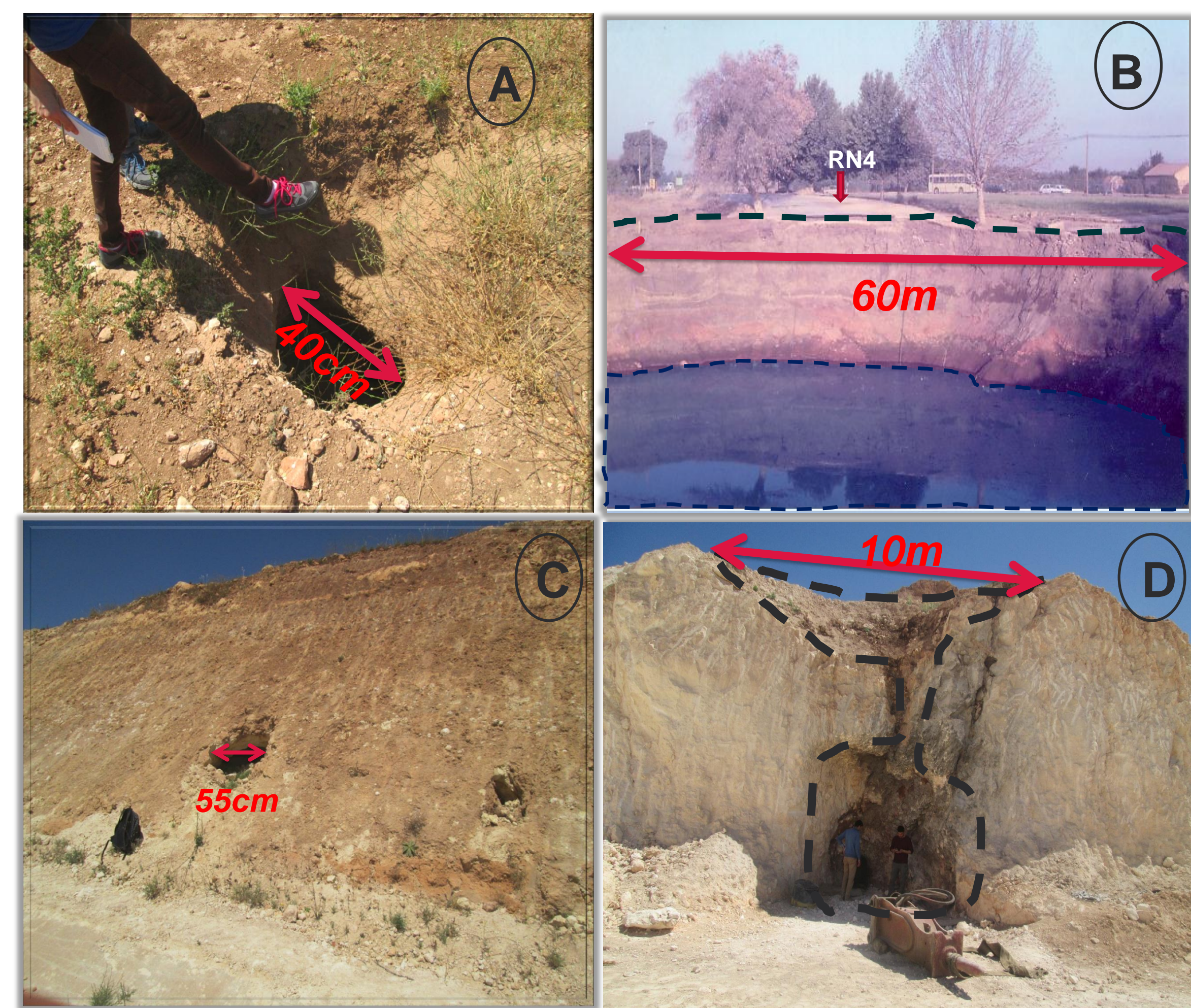
Fig.2: A) Sinkholes in study area; B) Sinkhole of the national road RN4 in 1988; C) Sinkhole in the quarry; D) Sinkhole near road.
