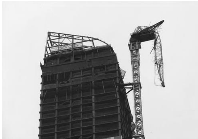
Figure 1. Crane failure in New-York, 2012 [1].
