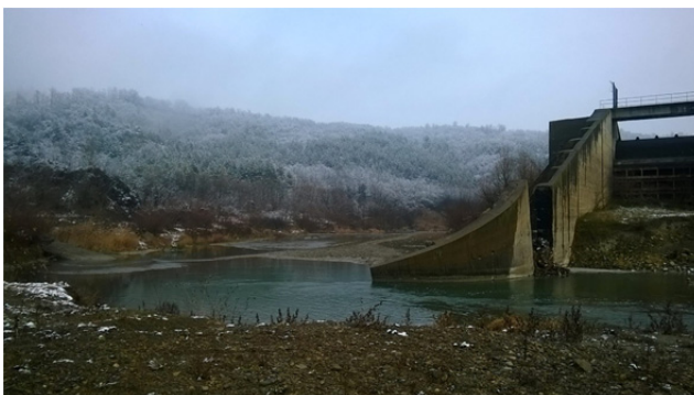
Fig. 2. The left bank of the Belci dam (Photo by Constantin Cristache, INCDFP, Romania)
