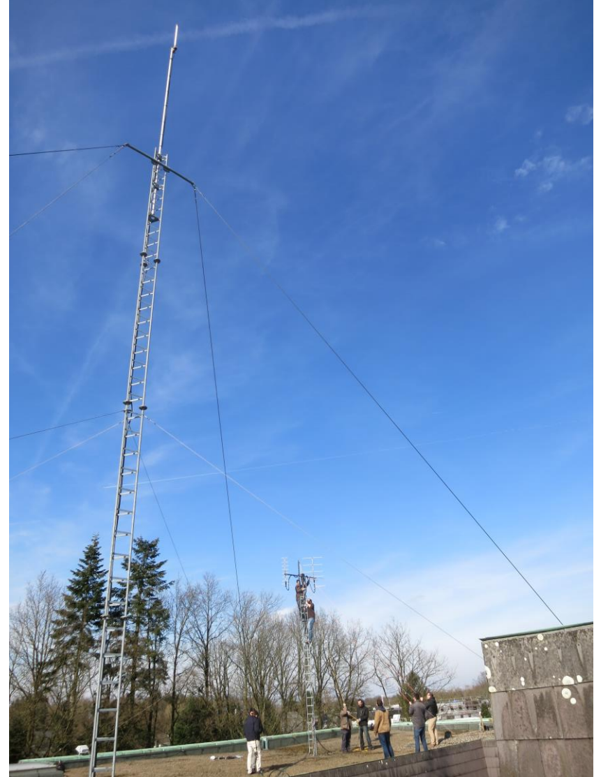
D-STAR repeater antenna
