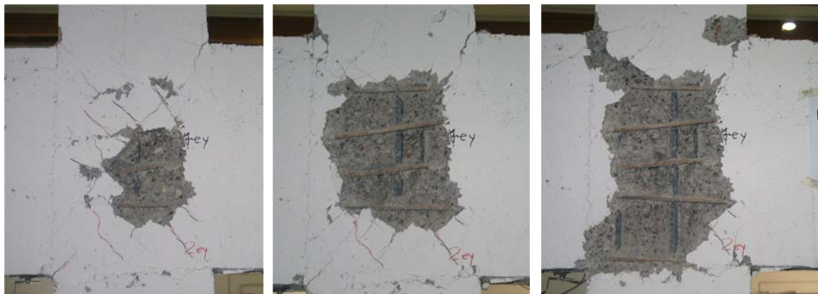
Figure 3-54. Pictures of the CO-Ts joint deterioration
