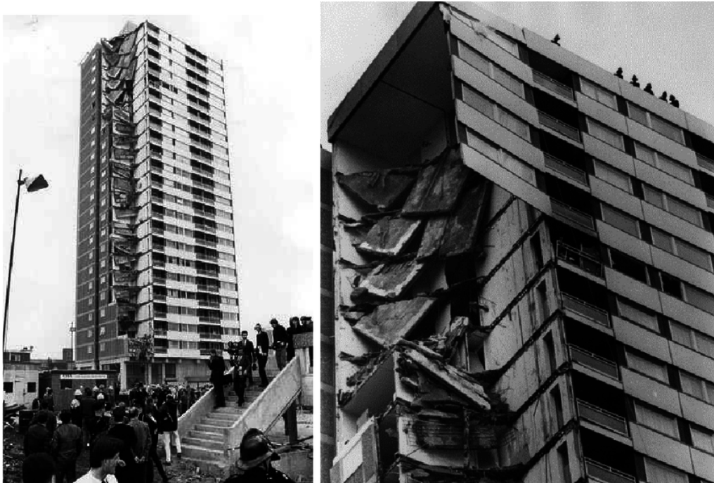
Figure I.1: Ronan Point apartment building progressive collapse (May 1968).
