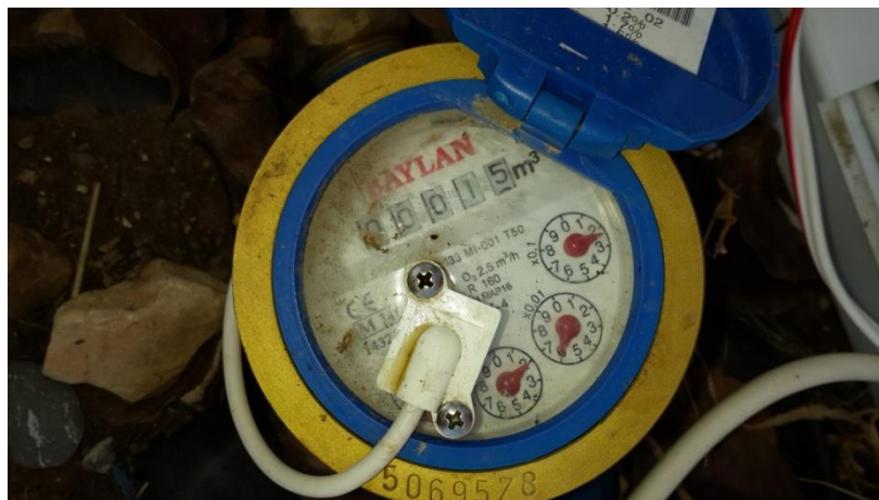
Fig. 3. Digital water meter
