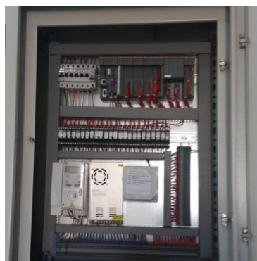
Fig. 1. IAS electrical panel
