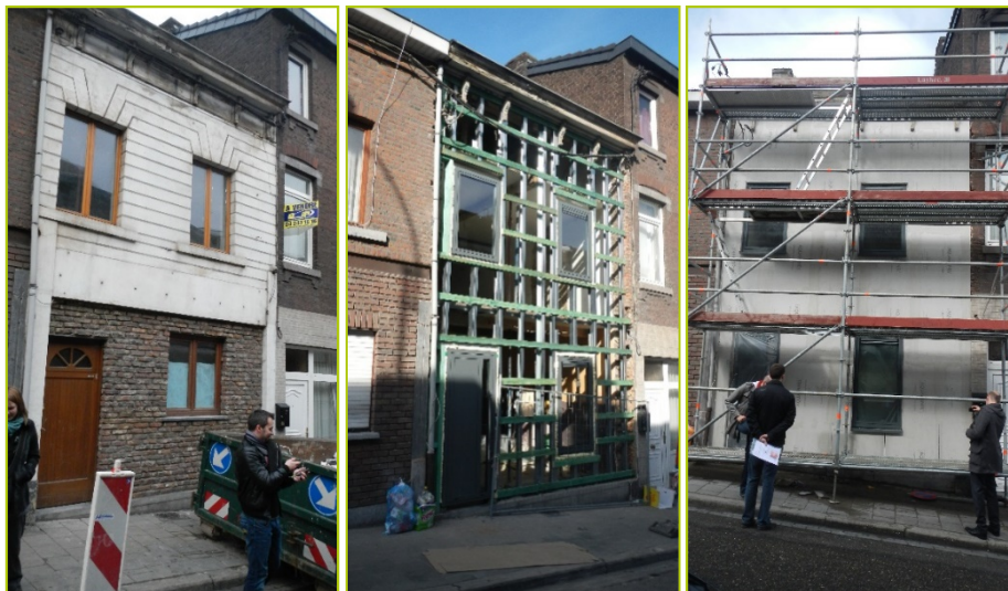
Figure 4. Facade of the building, before renovation (left), during structure erection (middle) and finishing covering (right).
