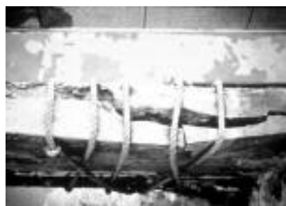
Extreme situation illustrating the need for repair engineering design and specifications (courtesy of the Structural Group, Columbia (MD), USA)
