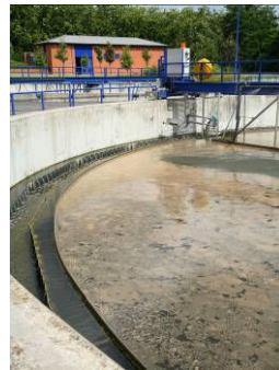
Separation between treated water and sludge Settling tank
