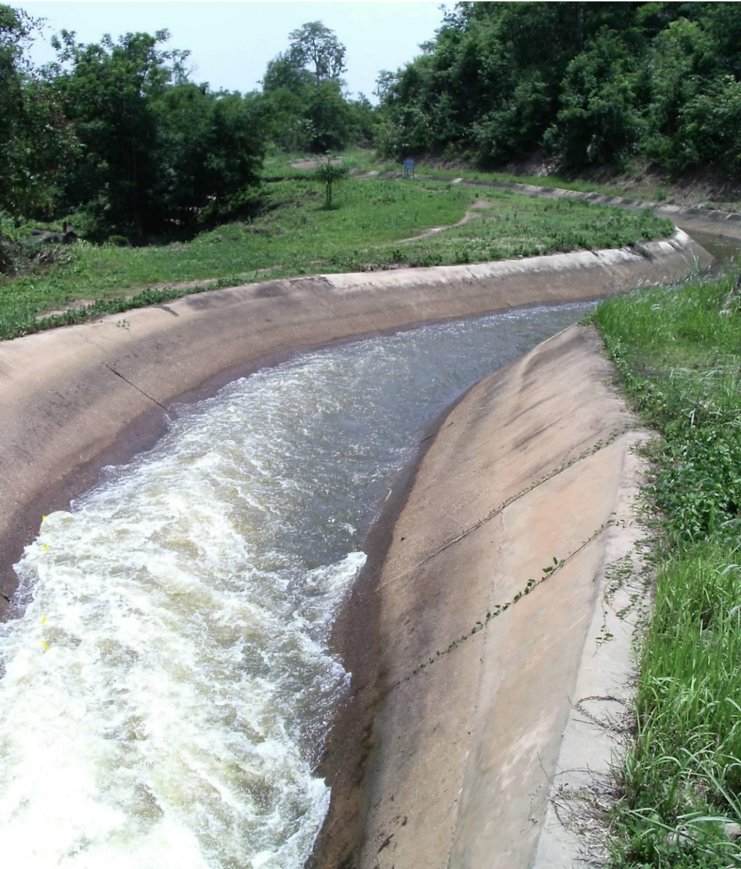
Concrete canal irrigation from the regulation pond of the Nam Mang 3 dam
