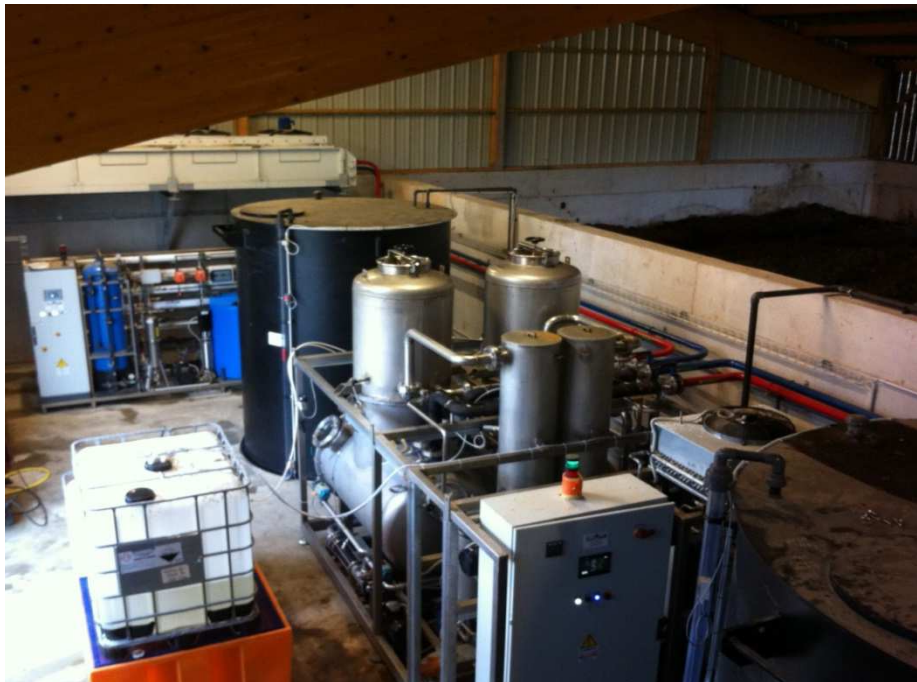
Figure 14: Treatment plant of digestate in the biogas plant “Pont Langlois”.
