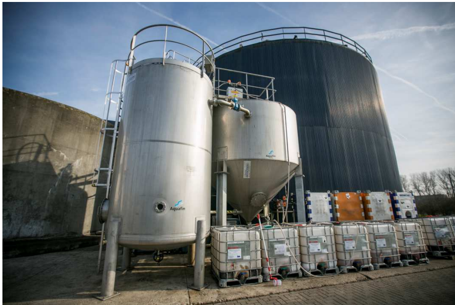
Figure 20: Picture of the pilot plant of struvite production designed by Aquafin.
