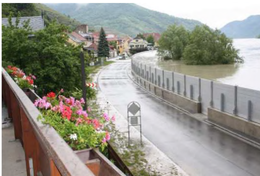
Mobile flood protection during the Danube flood in 2013 (© Provincial Government of Lower Austria)
