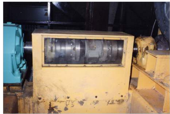
(b) Torquemeter between the electric motor and the mill shell.
