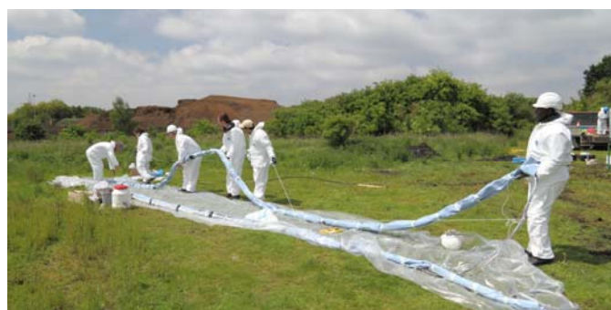
Figure 2: Flexible sleeve containing monitoring units
