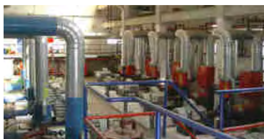
Figure 7 – Pump Station “A3” of Kozani District Heating
