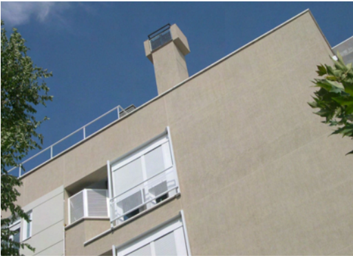
Figure 9 – New building. Natural chimney
