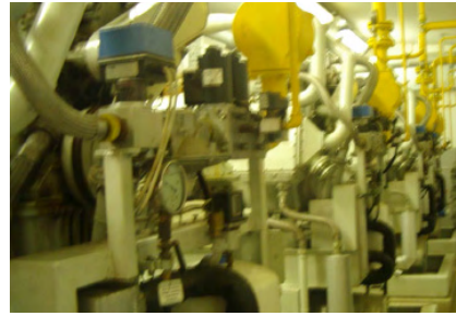
Figure 8 – Biogas engines in Noreikiskes power plant
