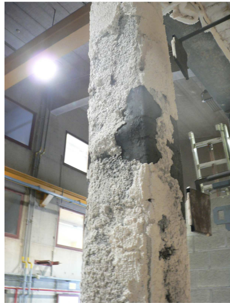
Fig. 3 Local buckling during test
