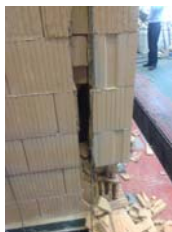
Figure 12. Collapse of the wall connection.
