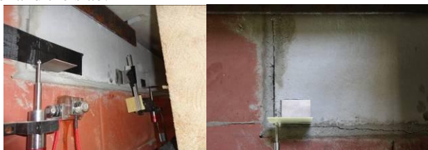
Fig. 6 – Cracking of the lintel
