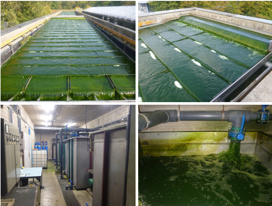
Figure 4.1: Top-left: light exposed part of the thin-layer cascade system on the roof. Top-right: zoom on the overflow tank. Bottom-left: engine room located downstairs. Bottom-right: zoom on a tank.
