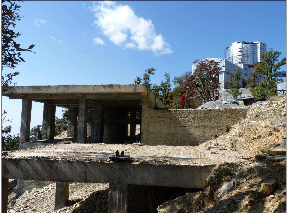
Figure 8.3: Present status of the ILMT enclosure along with the compressor room (front). The enclosure of the upcoming 3.6m DOT telescope is also visible in the background.
