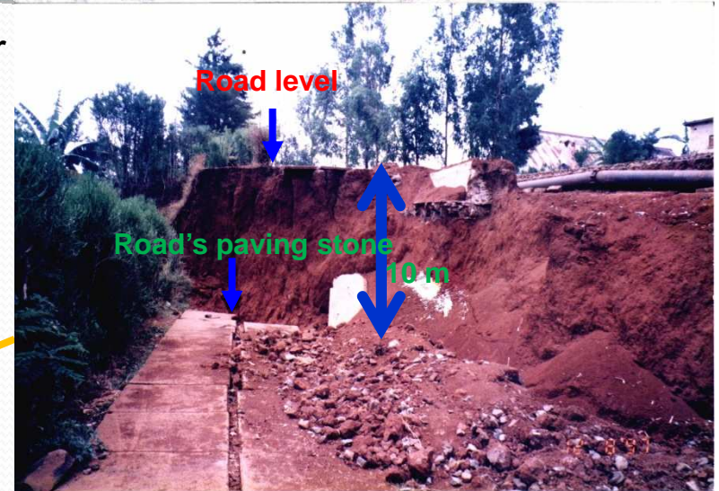
Figure 27: Landslide 1 day after event (12/8/1997)
