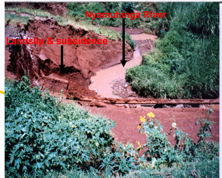
Figure 28: Landslide 1 week after event (18/8/1997)
