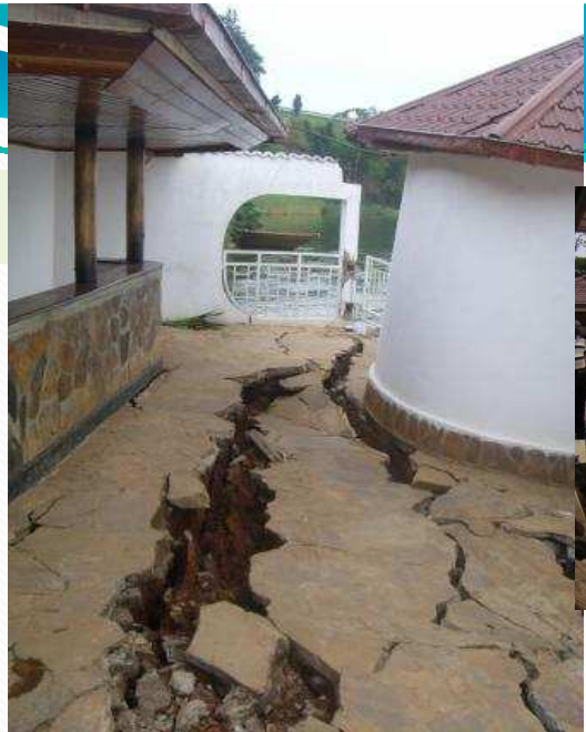
Figure 14: Subsidence at La Roche Hotel after the earthquake of 03/02/2008
