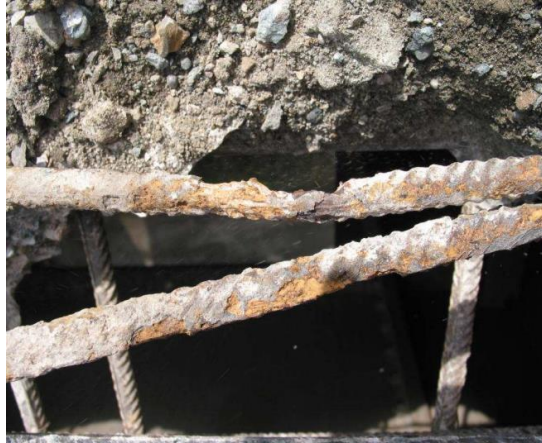
Figure 3 : Rebars corroded by a chloride contamination [9].
