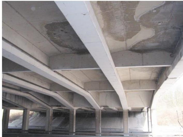
Figure 1 : Bridge deck suffering from concrete pathologies [9].
