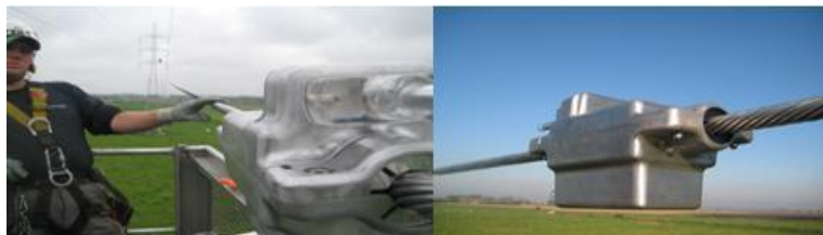
Fig. 2 Installation of the smart grids sensor Ampacimon on a 150 kV line in the north of Belgium, near the sea
