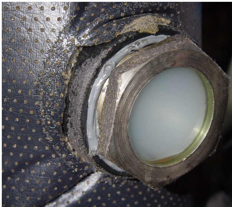
Figure 8.7. Oil fog visible in oil separator sight glass.
