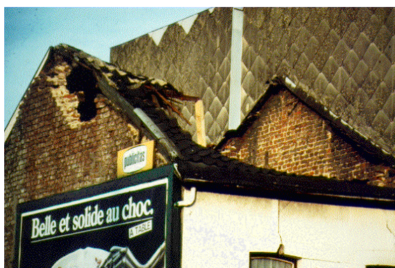
Figure 1 – Roof collapse during 1983 Liège earthquake
