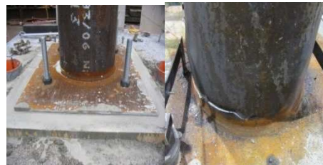
Figure 75.Innovative column-base joint for seismic loads: Geometry and Failure
