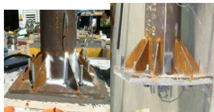
Figure 72. Standard column-base joint for seismic loads: Geometry and Failure
