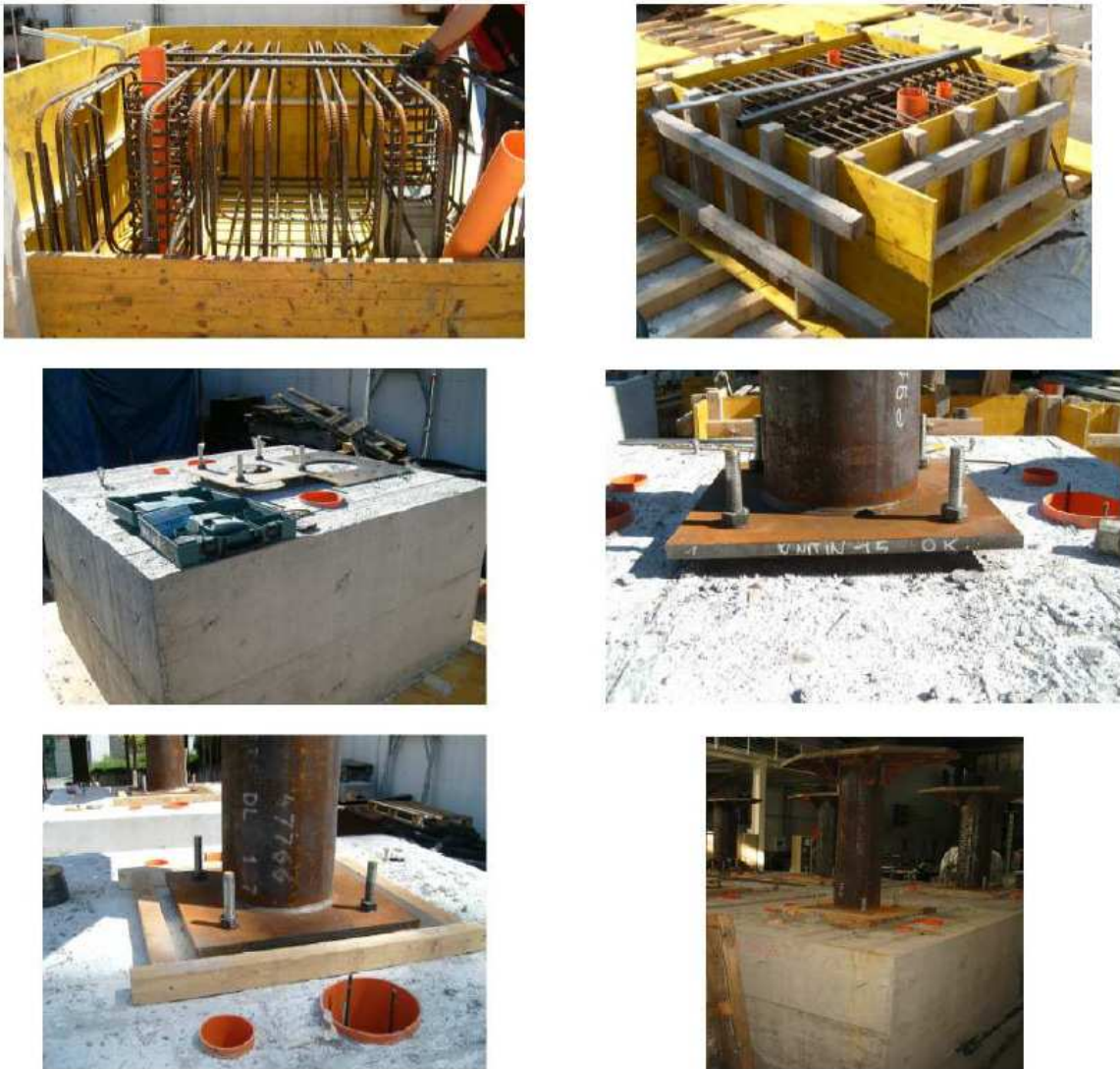
Figure 2. Realization of the column-base joints designed for the static solution at the UNITN Laboratory
