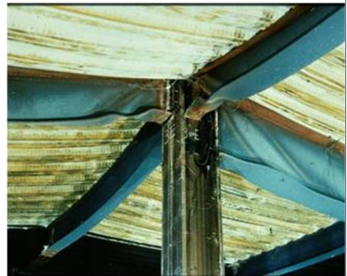
2 nd corner test: remaining deformed shape after fire
